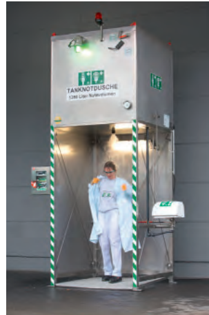
Tanknotduschen Tank safety showers
